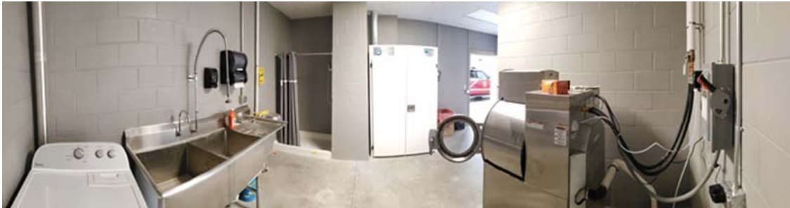
2 SMP design Inc.'s decon room for Madison Township (OH) Fire Station No. 183 includes a stainless steel double sink, washer extractor, gear drying cabinet, residential-style washer, and shower, with an access door to the outside.
