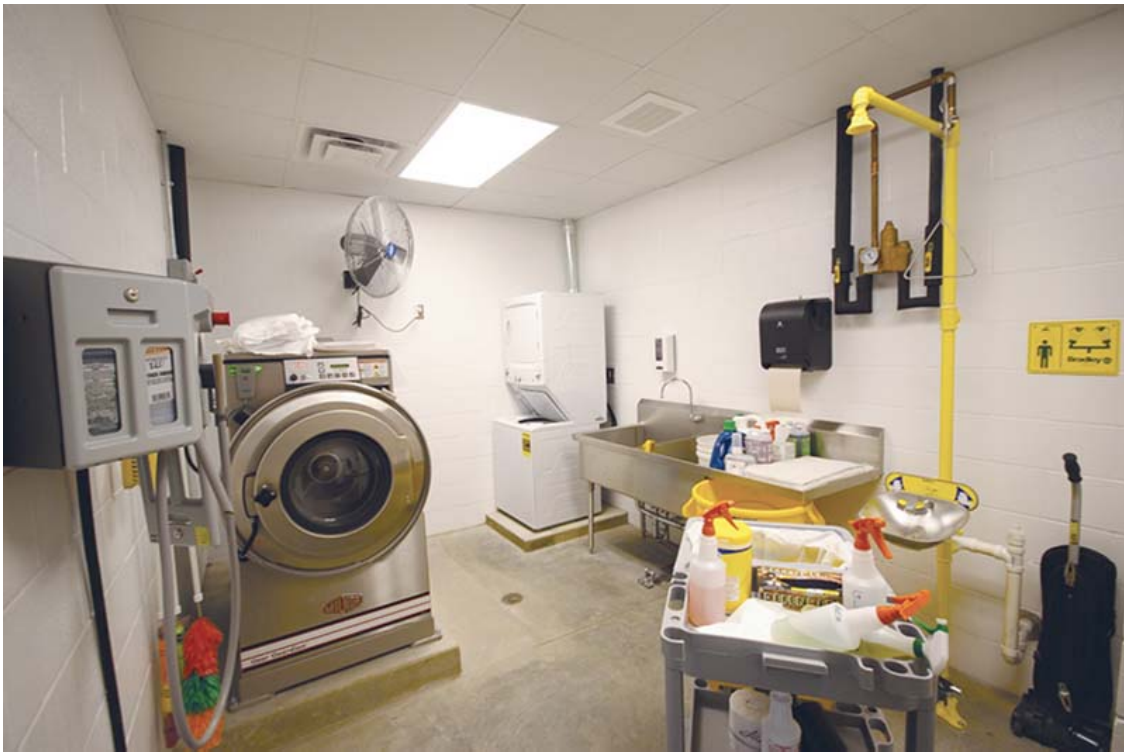
1 This decon room was designed by SMP design Inc. for Delhi Township (OH) Fire Station No. 36. (Photos 1-2 courtesy of SMP design Inc.)
